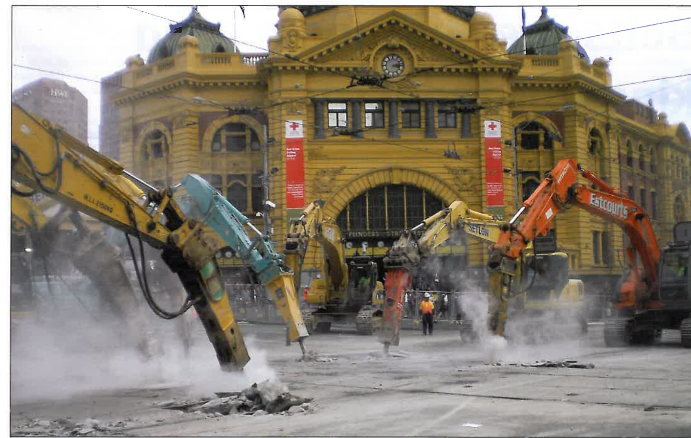
Altus put major diversions in place as excavators and hammers made short work of replacing tramlines at Melbourne's busiest intersection outside Flinders Street station, during Easter 2008.
